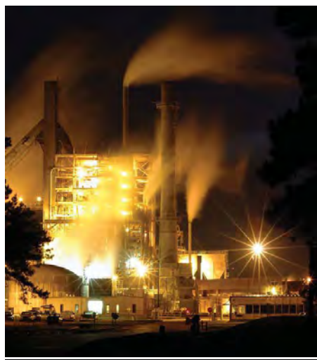
Figure 5: Like most pulp/paper mills, International Paper Company’s mill near Pineville, La., burns bark and wood waste in its boilers to generate both heat and electrical power.
